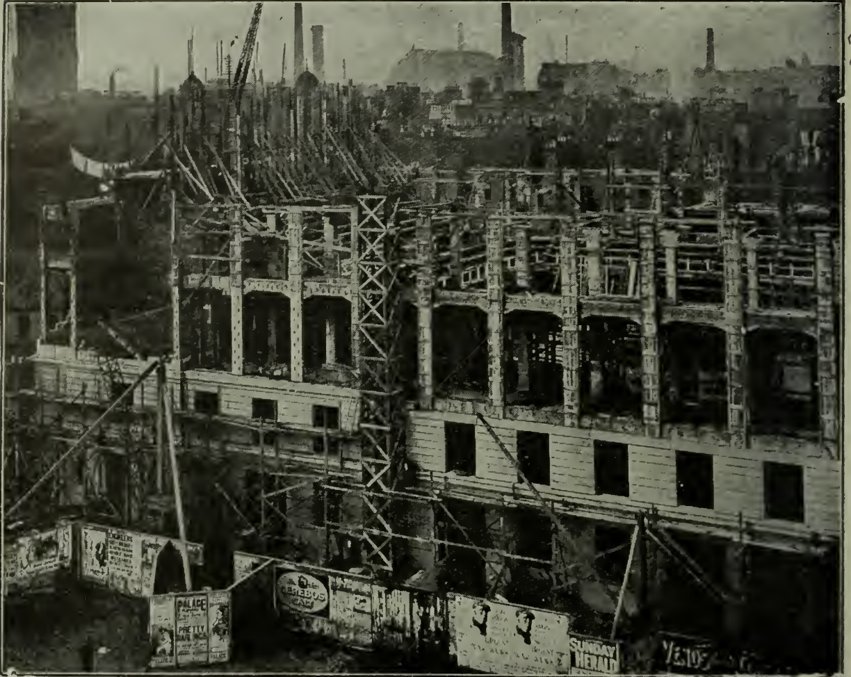
City Hall, Dundee, in course of construction. Pile Foundations & Ferro-Concrete Superstructure executed by us.
